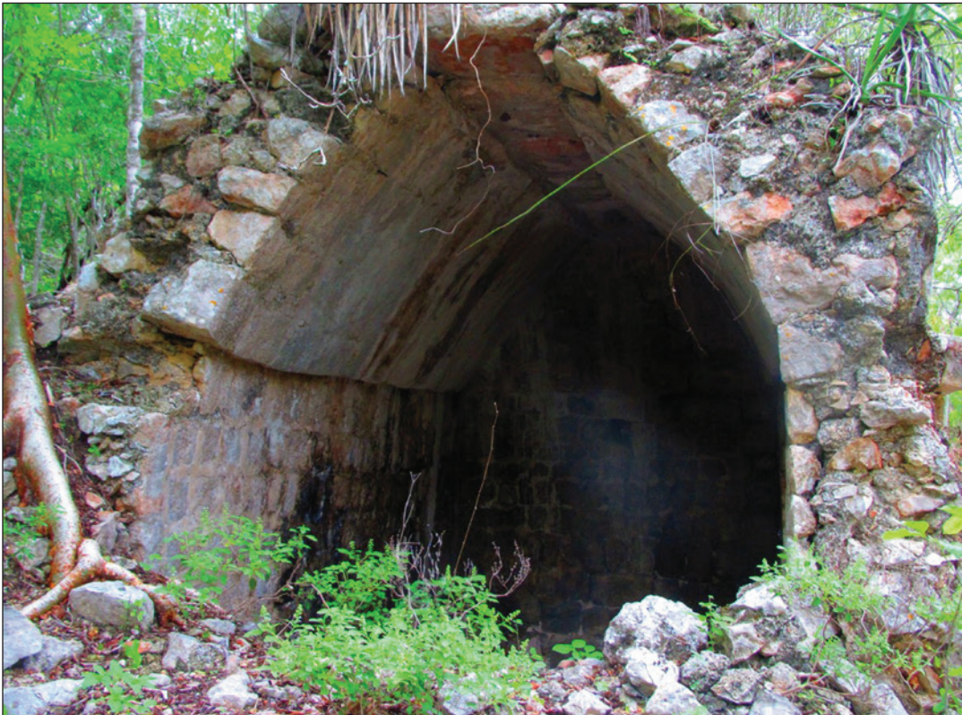
Figure 3. Photo of a partially collapsed vault at the site of Kiuic showing the amount of lime mortar that would have been necessary to construct these buildings (photo by author).
